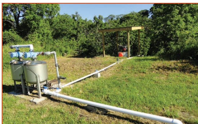
Figure 7. A sand filter (foreground) filters creek water delivered with a gas-powered pump (background).
