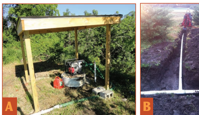
Figure 8. (A) A gas-powered 10 hp pump is covered to reduce wear from environmental damage and keep the engine cool during operation. (B) Belowground 3-inch PVC piping distributes water to various production fields.
