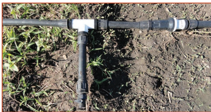
Figure 6. High pressure (50 psi) is maintained to distribute water with a pressure regulator (right) installed at the beginning of the header pipe. A garden hose thread connector at the end of the “T” allows for watering and overhead irrigation.
